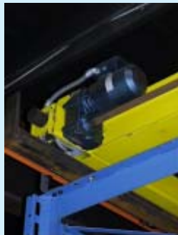
Geared Drive For Bridge Movement Via VFC Motor Controllers
